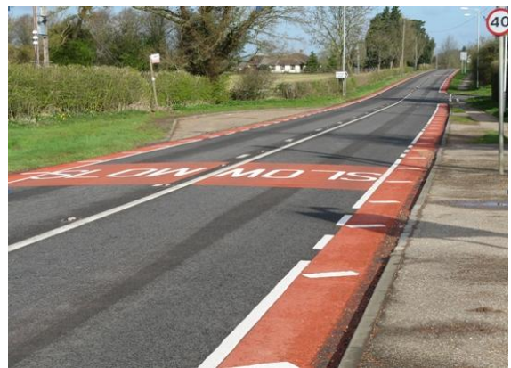
Red markings on Welford Road (A 5199)
